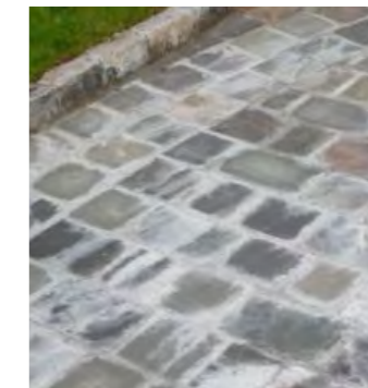
Cement staining on setts
