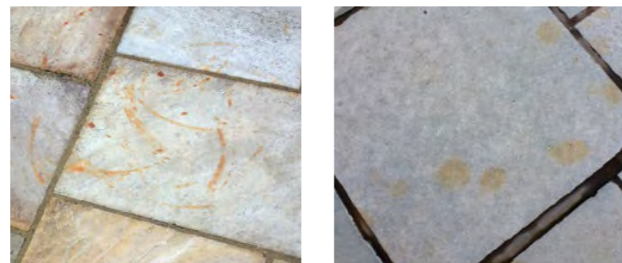
Rust stains from patio furniture
